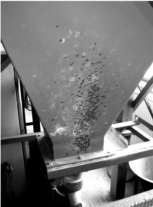
Fig. 1.1. Traces of hammering at a hopper wall indicating flow problems
