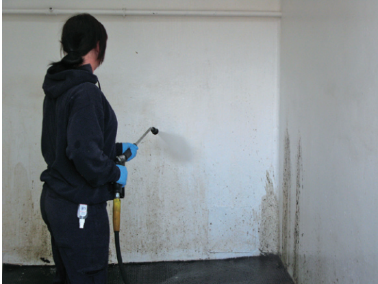
Fig. 1.9 Hot water or steam and chemical solutions under pressure can be used to improve the disinfection of a stable, where an infectious agent might have been present.
