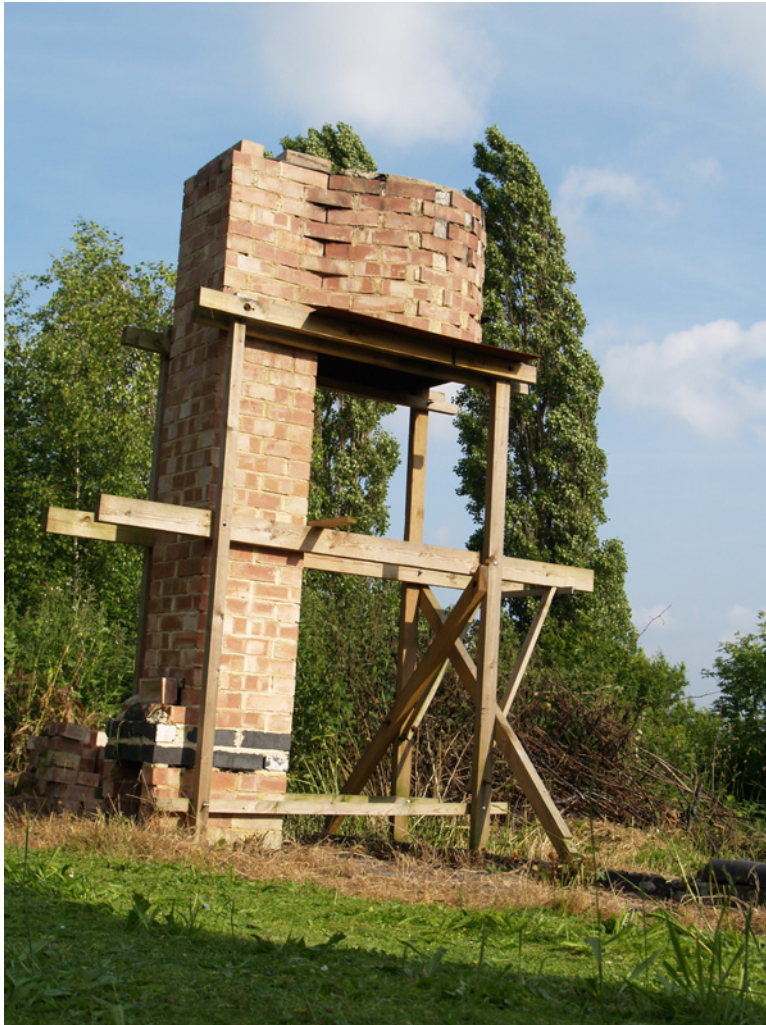
Figure 1.1 Furnace, flue and upper displacer cylinder re-constructed full-size to the drawings and dimensions of the Edinburgh patent
