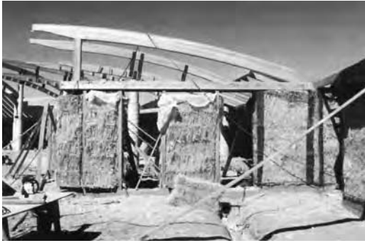
Fig. 1.8 Construction phase photo of Real Goods Solar Living Center straw bale walls. Design intent becomes reality during this phase. (Reprinted from A Place in the Sun with permission of Real Goods Trading Corporation.)
