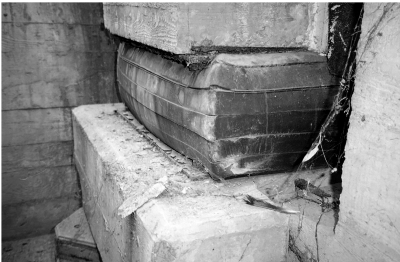
Figure 1.4 Unreinforced bearing in the Pestalozzi school building in Skopje. Courtesy of James M. Kelly, NISEE Online Archive, University of California, Berkeley
