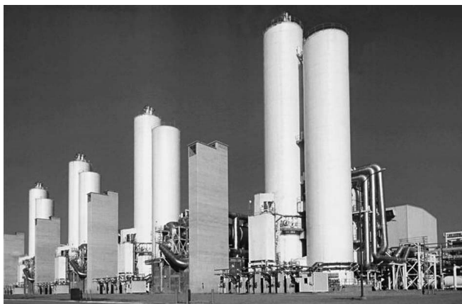
Fig. 1.3 Air separation unit at Cantarell, Mexico (2000).
