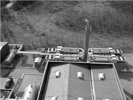
Figure 1.3 Combined heat and power plant in Dortmund/ Derne with four modules for G.A.S. Energietechnologie GmbH (order value approx. 3 million €).
