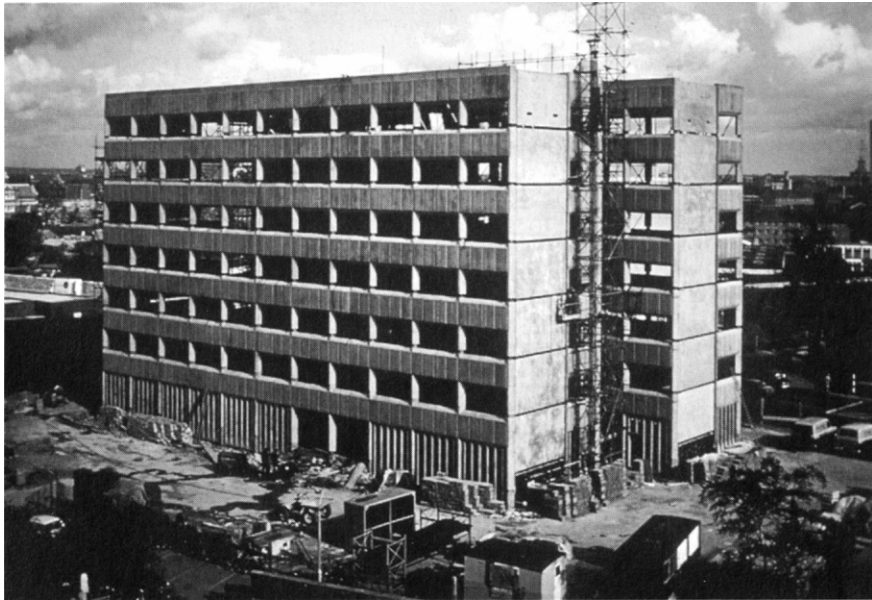
Figure 1.4 Precast construction of the 1960s using the National Building Frame, The building is Highbury College, now part of the University of Portsmouth (courtesy of Costain Building Products).
