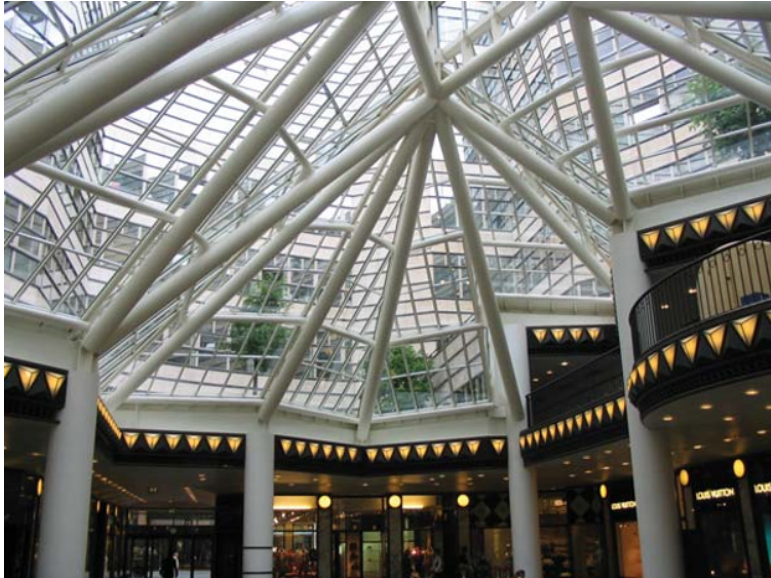
Fig. 1.2 Roof structure of Quartier 206 shopping mall, Berlin. Quite a ‘muscular’ roof structure!
