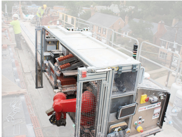
FIGURE 1.1 Automated construction of an architectural wall. If the craft isn't in the assembly in the field, where does it lie? In the programming of the automation?
